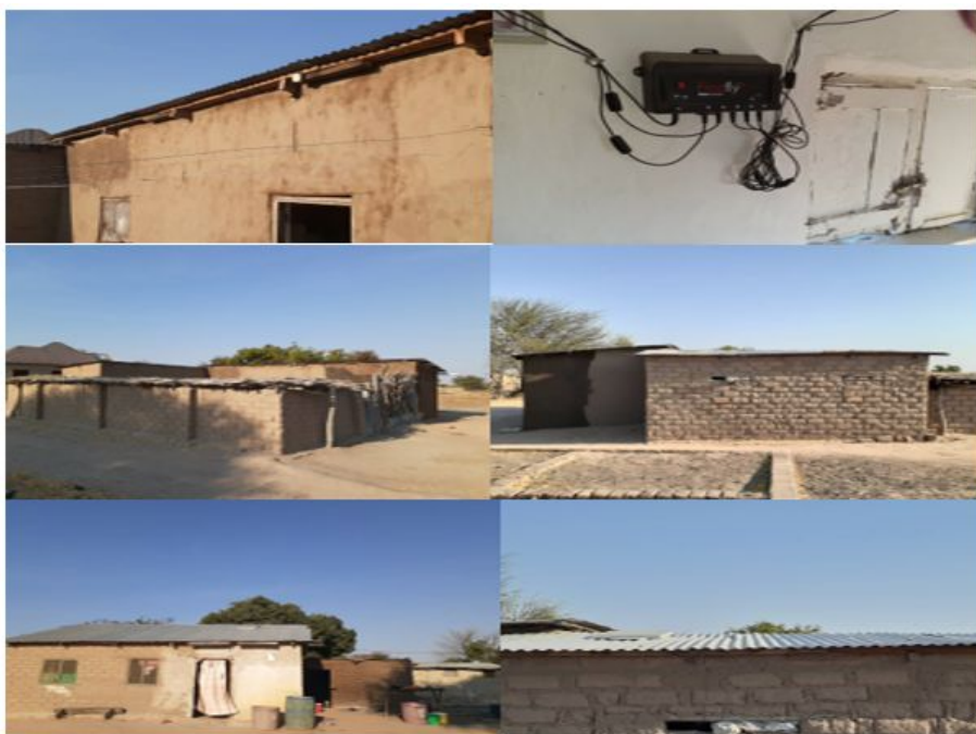
📷 Household solar energy installation, Makutopora village in Manyara, August 2019. Photo: Hannington Muyenje/Tearfund
