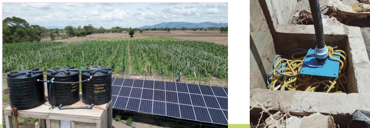
Figure 15: Three Interconnected water tanks with 2 inches pipe and borehole casing cap
