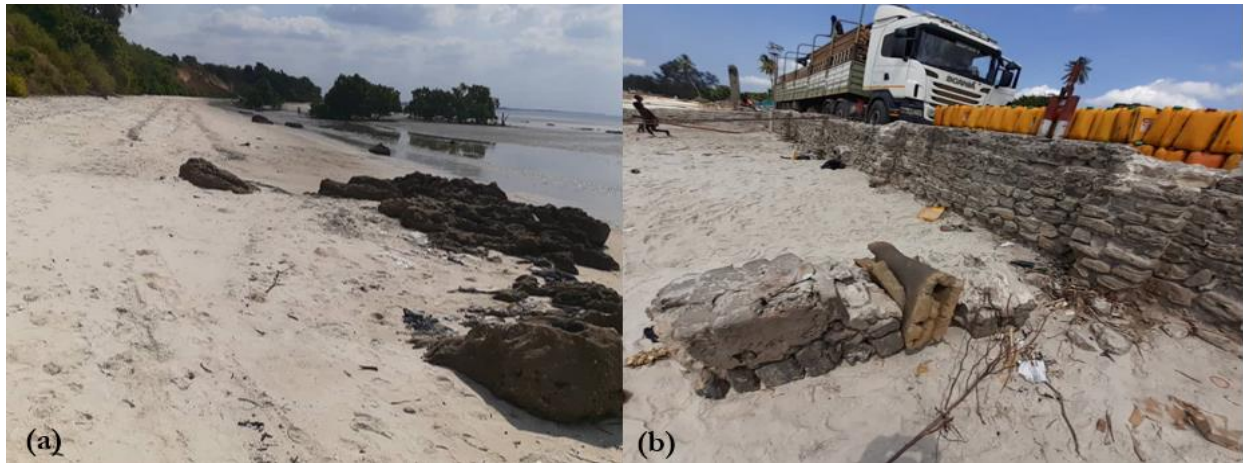
Figure 21: Evidences of goods and services loss and damages in Bagamoyo district
